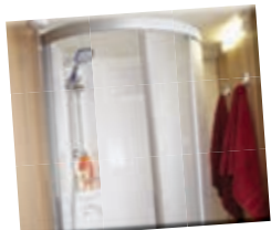
Circular shower cubicle
